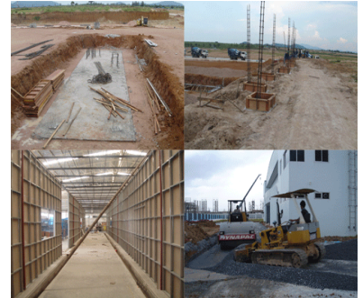
Photos of the China State Bank public housing development construction site managed by Knight Industrial Services Co, Ltd. Thailand
